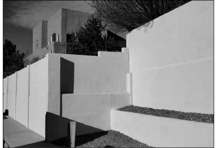
These photos (left and right) show the brand new stucco walls in High Desert following recent repairs.
